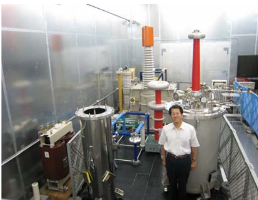
Cryogenic high-voltage laboratory
